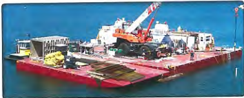
A barge and dive station was set up for work on the Auxiliary level intake at Cheesman Dam and Reservoir. The materials barge moored alongside provides temporary storage for sections of a removed trashrack and a stainless steel spool being prepped for installation.
